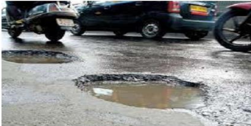
Figure 1 Condition of roads with potholes [1].
