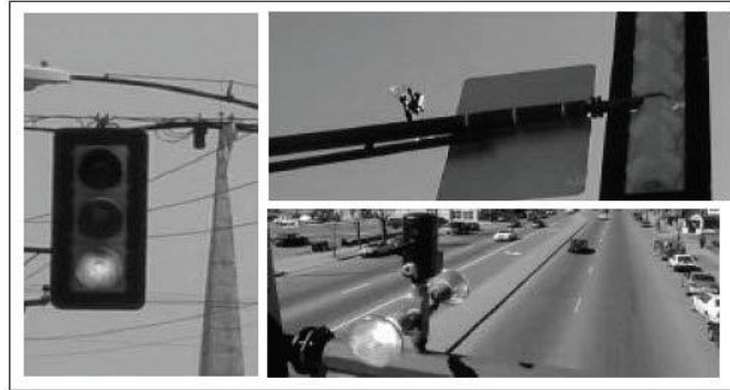
Figure (iii) Traffic Signal Mast Detector and Indicator Light
