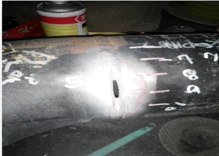
Fig 1. Pipeline Showing Crack with Measurement (Picture Courtesy- SADARA, KSA)
