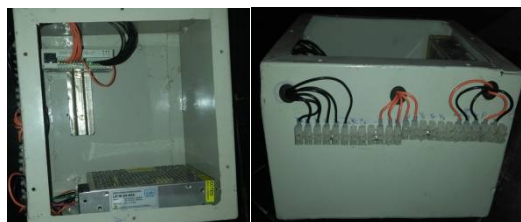
Fig 5 Overall Control Panel
