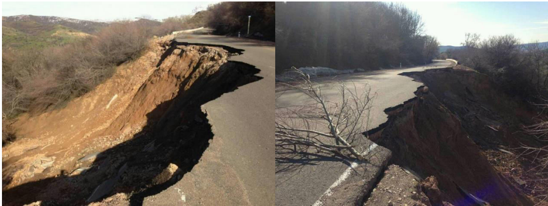
Figure 1. Landslides on the area of the road Tashkent – Chimgan, (March, 2017y.)
