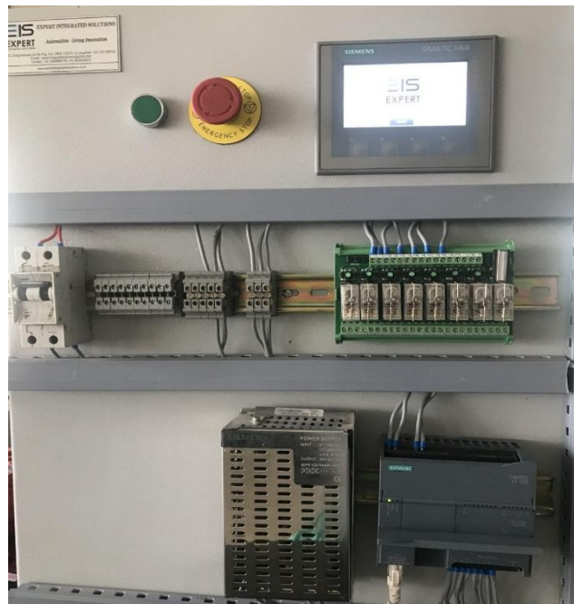
Fig 7: Smart gear finishing machine by Expert integrated solutions Ltd
