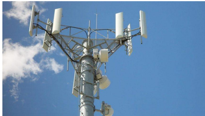
Figure 1: Antenna Array under LTE Network
