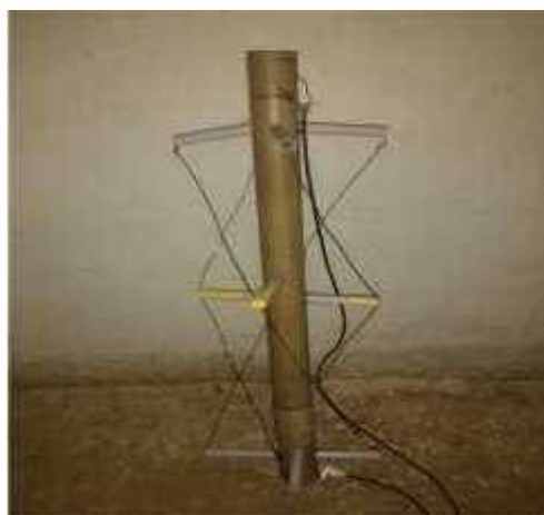
Figure 3 Open air mounting of the radio wire
