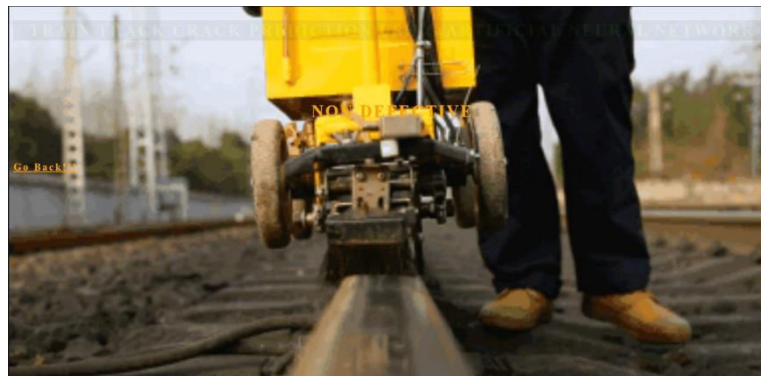
Fig 7: Crack not detected
