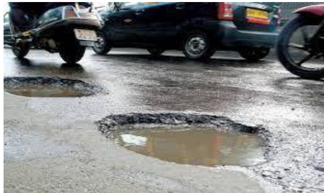
Fig. 1. Condition of roads with potholes.
