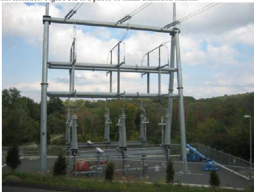
Figure.3.2 Small transition station.
